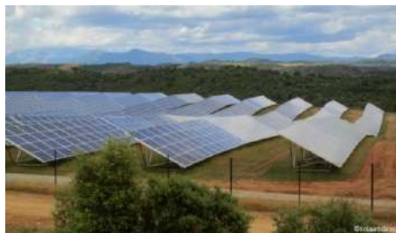
Figure 10: parc photovoltaïque au sol (source BayWa r.e. France)
